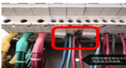
28#楼4F走廊两路线过热烧焦
